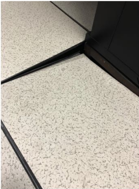
Gap between the tiles
